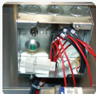
Inside the junction box. (Pictured: door activation switch)
