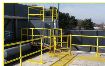
ROOF FALL PROTECTION RAILING
