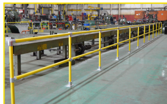
WALKWAY GUIDE RAIL
